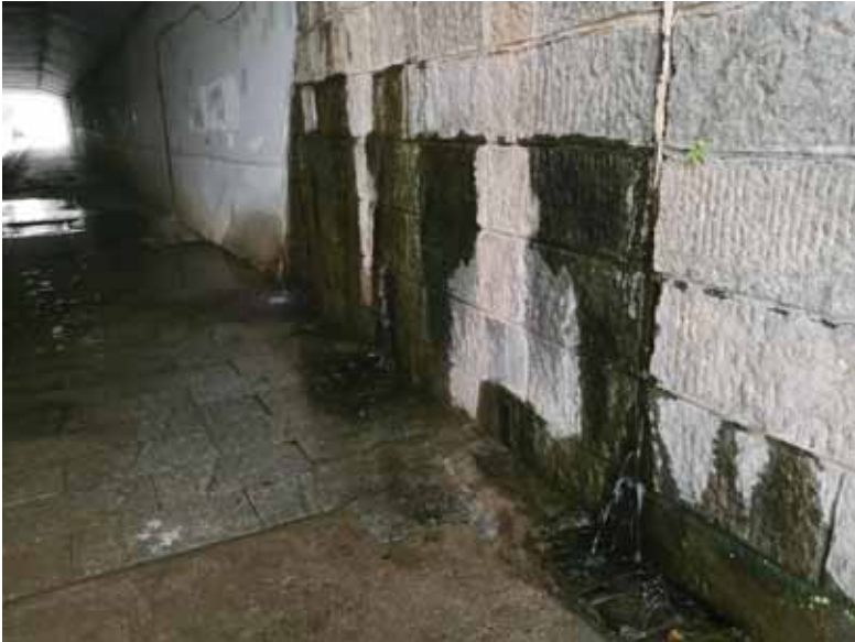
涌水洞孔墙体上布满青苔
